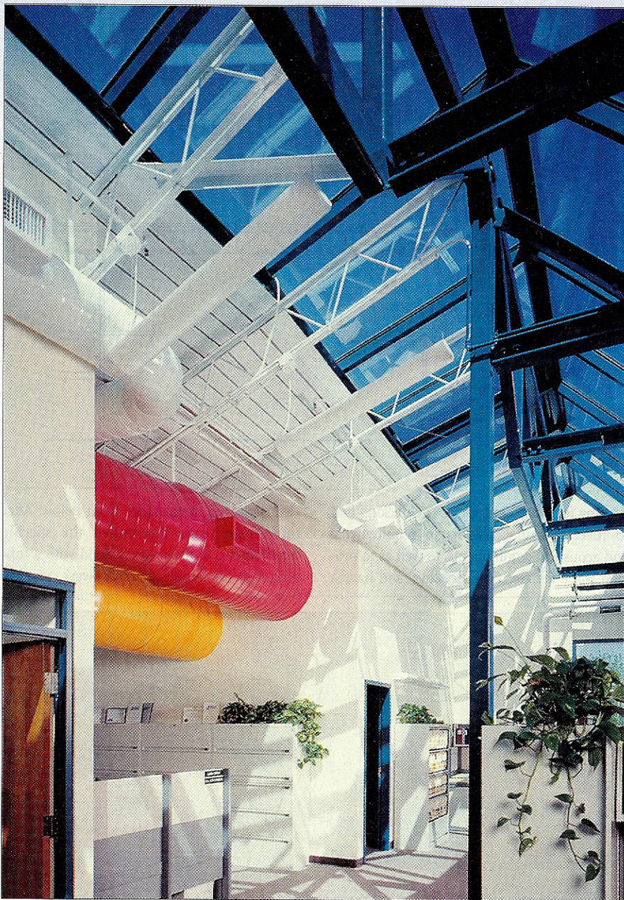
The exposed mechanical ducts and steel joists result in a light, airy interior office space.
