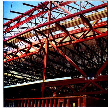
An inverted chevron braced frame is blended into a typical girder truss.
